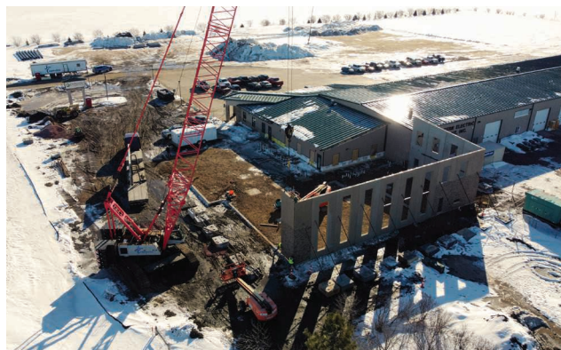
Progress continues to be made on the expansion at our Sioux Falls office.
