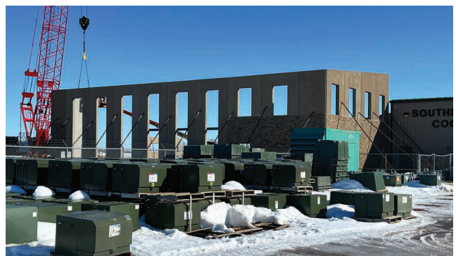
Pre-formed walls are being set-in-place and hope to have all the walls set in a couple of weeks
