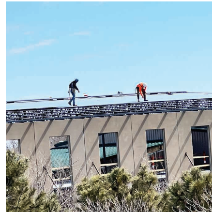
Progress is being made on the second story roof at the Sioux Falls office expansion.
