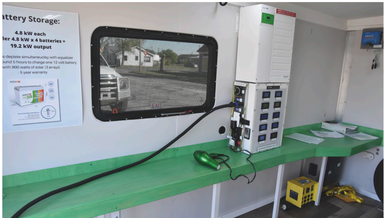
The interior of the solar trailer is equipped with battery storage and outlets – powering everyday electrical appliances, such as a hairdryer.
