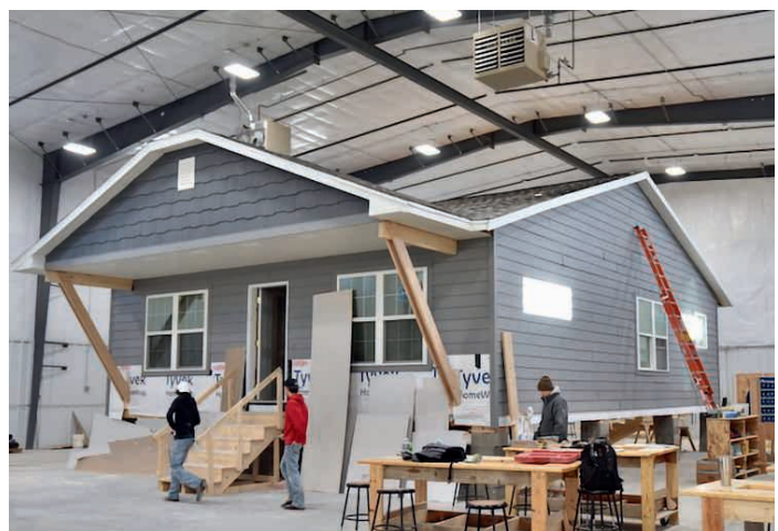
Students in the Harrisburg School District's home builders academy have built a full house. Photo courtesy of John Klemme
